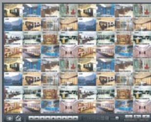
central monitoring system (CMS)
